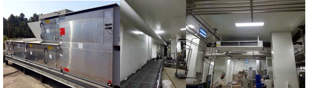
Bonjus AC and Contamination Control For Ice Cream Production Room Fonar Beirut Lebanon (2015)
