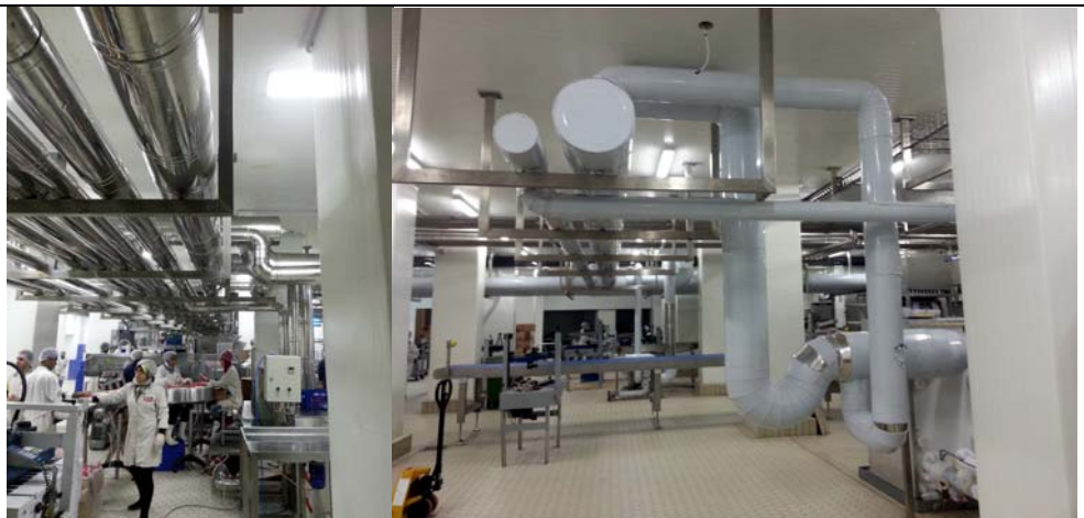
Bonjus Ammonia Plant Upgrading 315kW -45°C 175kW -35°C 876kW -10°C Fonar Beirut Lebanon (2015)
