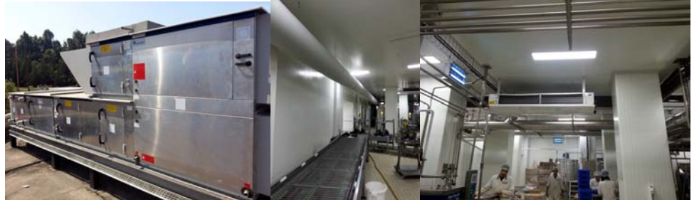
Bonjus AC and Contamination Control For Ice Cream Production Room Fanar Beirut Lebanon (2015)
