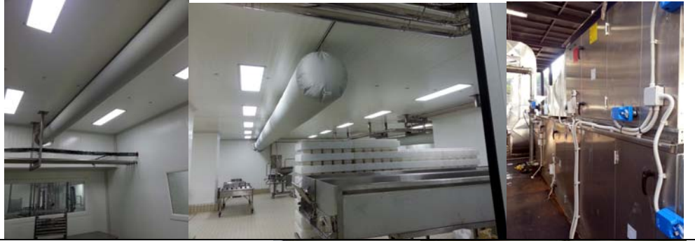
Taanayel Les Fermes Cheese Factor AC and Contamination Control System for Production Rooms Fanar Beirut Lebanon (2015)
